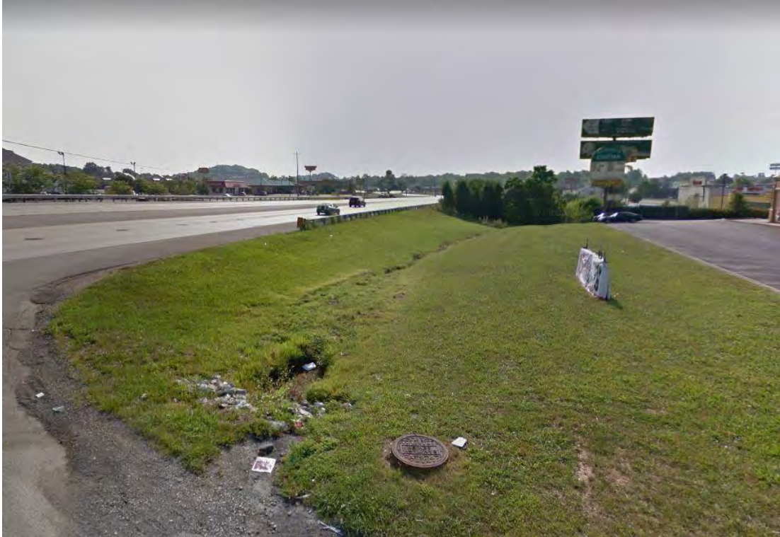
Figure 23. (Point A). Drainage along south side of KY 192 at intersection of Oscar Barnett Drive and KY 192.
