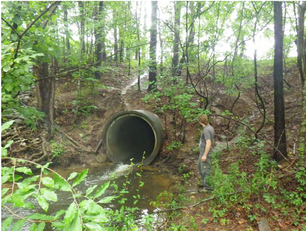
Figure 19. View to west of drainpipe in drainage to southeast of post office.
